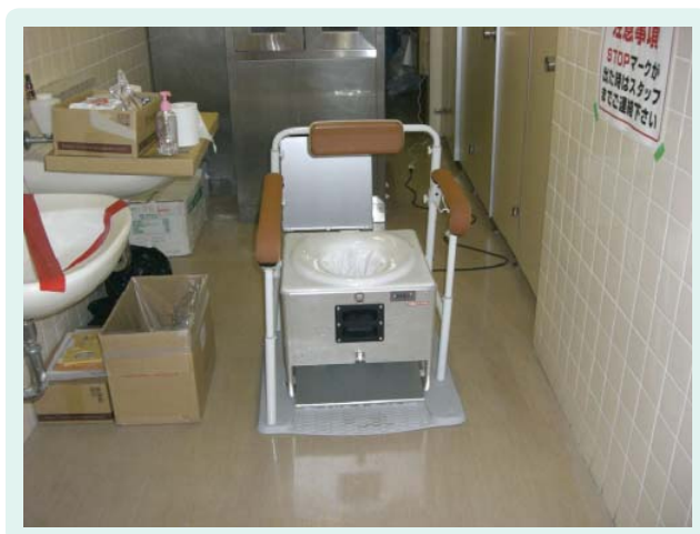
Figure 2. Wrap-type toilet used in evacuation centres
